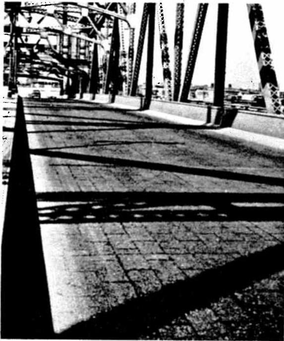
Fig. 8.10. Asphalt plank wearing surface on the Harlem River Lift Bridge, New York City
