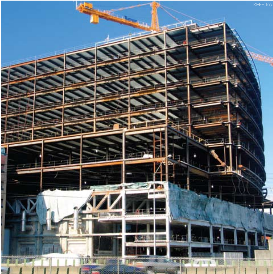
Providence Portland Medical Center Portland, OR Constructed 2006
