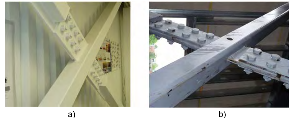
Figure 1. Bolted connections at brace intersection in X-bracing: a) Single shear lap splices; b) Double shear lap splices.
