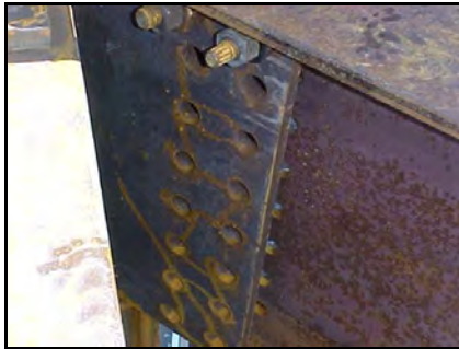
Figure 1: Misaligned bolted shear tab connection requiring retrofit (courtesy of DPHV)
