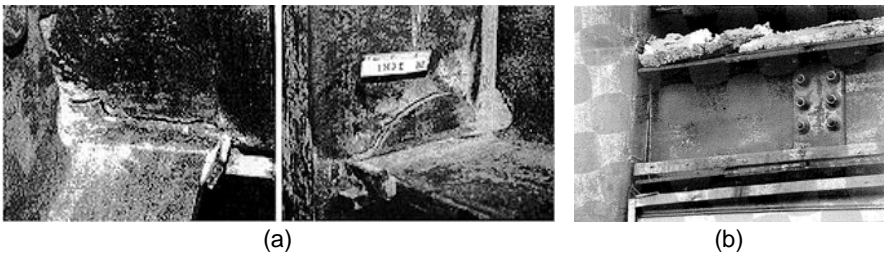
Fig. 2 Failure of the beam-to-column welded connections: (a) Northridge earthquake; (b) Kobe earthquake
