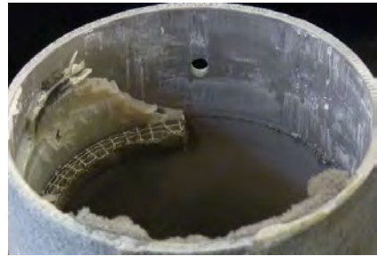
Figure 10b: Fracture appearance outer tube (Ummenhofer et al. 2015)
