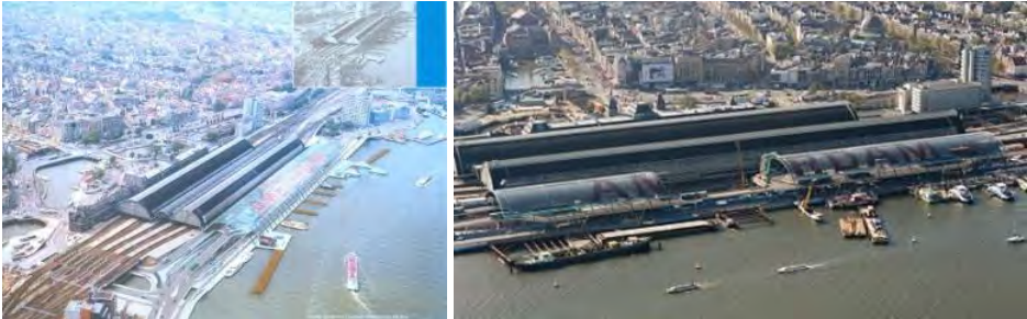
Figure 8. Artist impression of the extension Railway Station Amsterdam with the glass roof under construction (April 2012, project JSEI).
