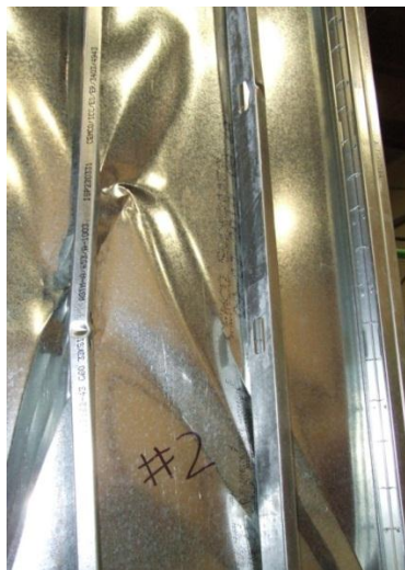
Figure 8: Distortion of interior studs
