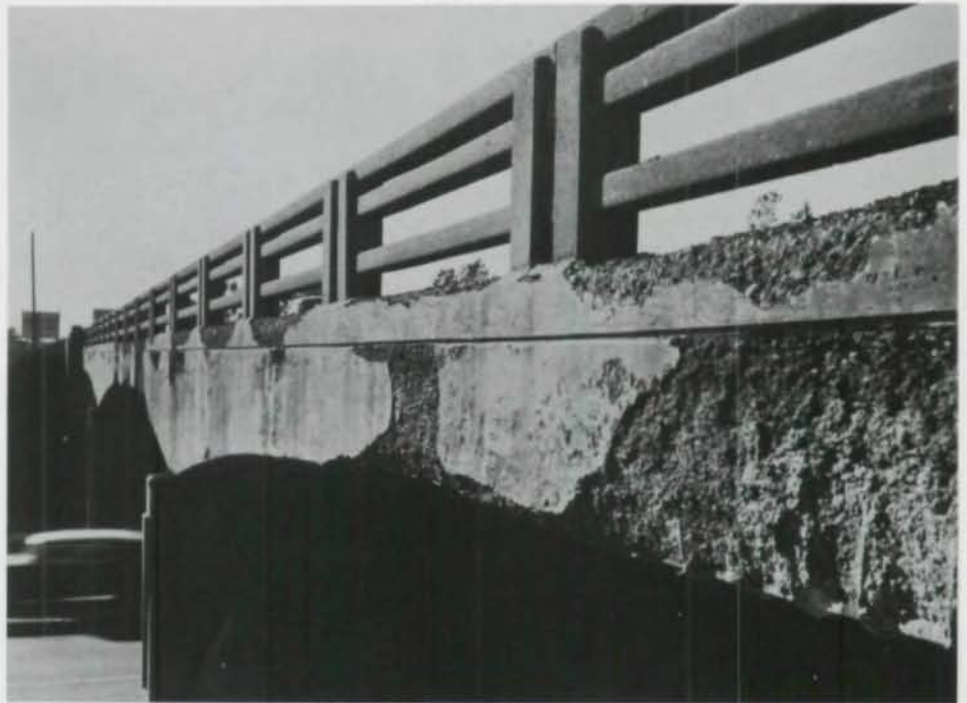
As may be seen 20 years of de-icing chemicals have taken a toll on this concrete bridge. Severe spalling has created hazards for motorists when chunks of concrete have fallen unexpectedly into the streets below.
