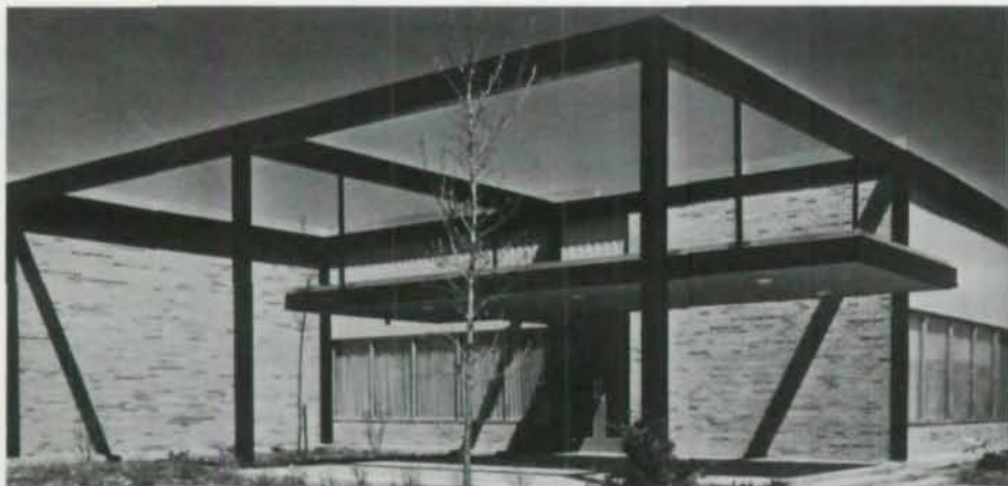
Structural steel framework for Globe-Union is wide-flange exterior columns, five-inch pipe interior columns, wide-flange beams, and open webbed joists five feet on center.
