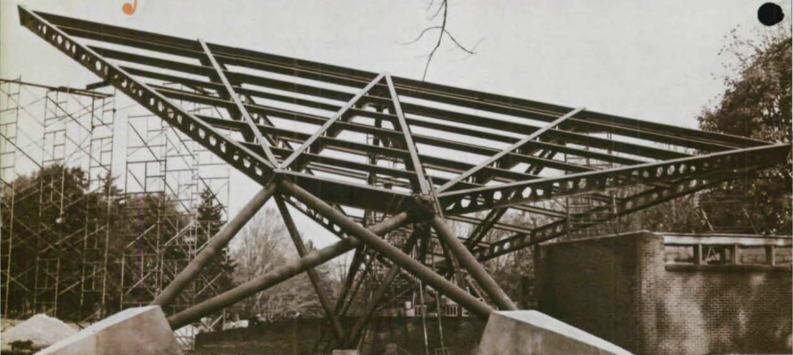
The free-standing roof of the Sertoma Band Shell is like a square that has been folded on a diagonal, with one peak tipped up, and its "wings" clipped.
