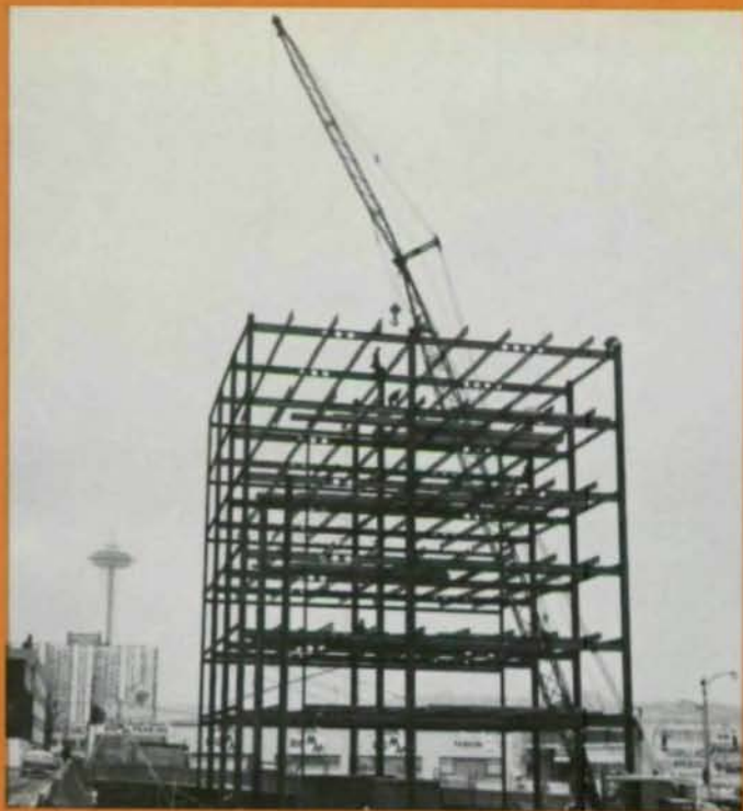
Steel framing for the first six floors of Seattle's 6th & Lenora Building was erected in less than a month. Note web holes located at midspan where shears are low.
