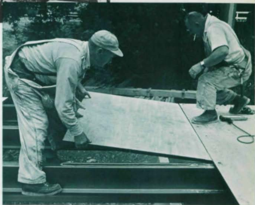
These 1 3/8-in.-thick plywood panels are easily dropped into place on steel floor beams. New adhesive simplifies wood-to-steel connections.
