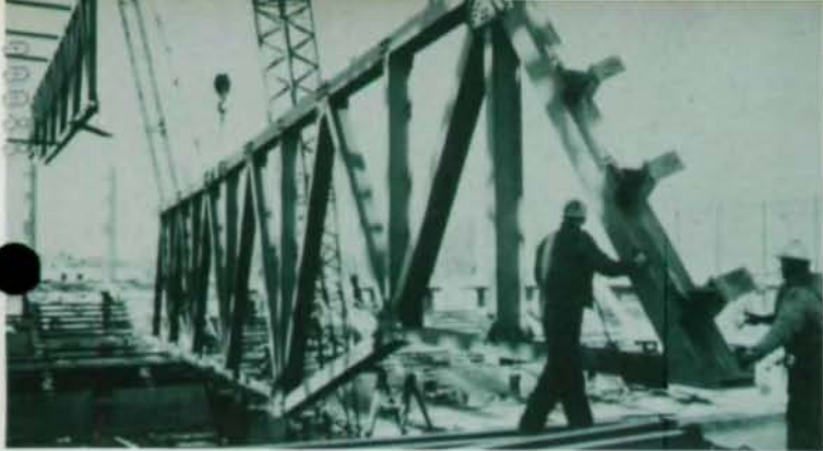
Scaffolding provides work platform 58 feet off ground for erection of 97-ton truss over arena.
