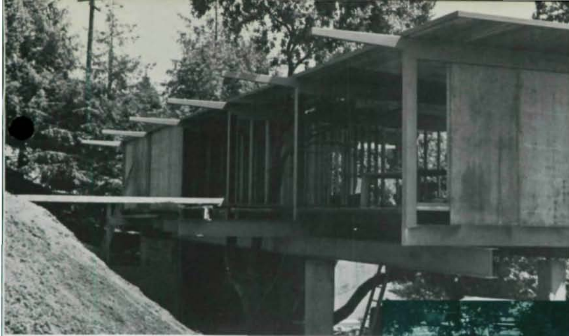
Two wide-flange steel beams span 40 feet between supports and cantilever 18 feet beyond, providing carport area. Attractive steel footbridge, replacing plank shown at this stage of construction, serves as main entryway to house.
