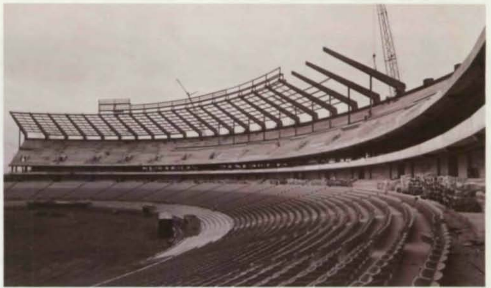
Steel construction leaves no spectator behind a post on either grandstand level.
