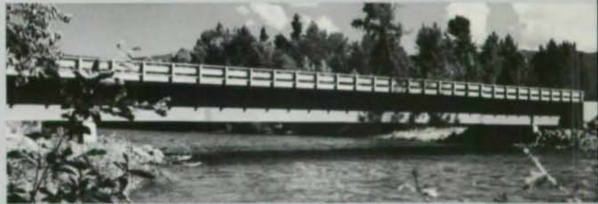
AWARD OF MERIT – SHORT SPAN Cle Elum River Bridge, Kittitas County, Washington Designer: Arvid Grant & Associates, Engineers Owner: Kittitas County, Washington General Contractor: Anderson Bridge Company Fabricator: Union Iron Works Division—Coeur d'Alenes Company
