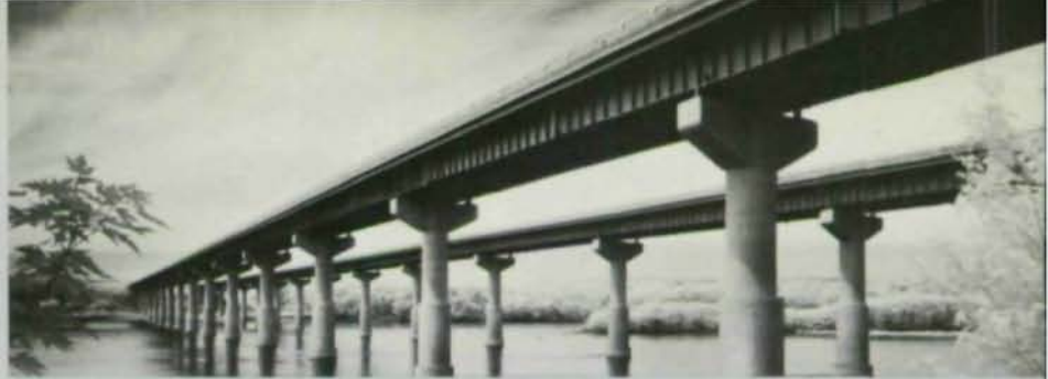
AWARD OF MERIT – MEDIUM SPAN, HIGH CLEARANCE Mifflinville Bridge Over The Susquehanna River, I.80, Columbia County, Mifflinville, Pennsylvania Designer: Brookhart & Tyo, Consulting Engineers Owner: Pennsylvania Department of Highways General Contractor: Woelfel Engineering Corporation Fabricator: Harris Structural Steel Company
