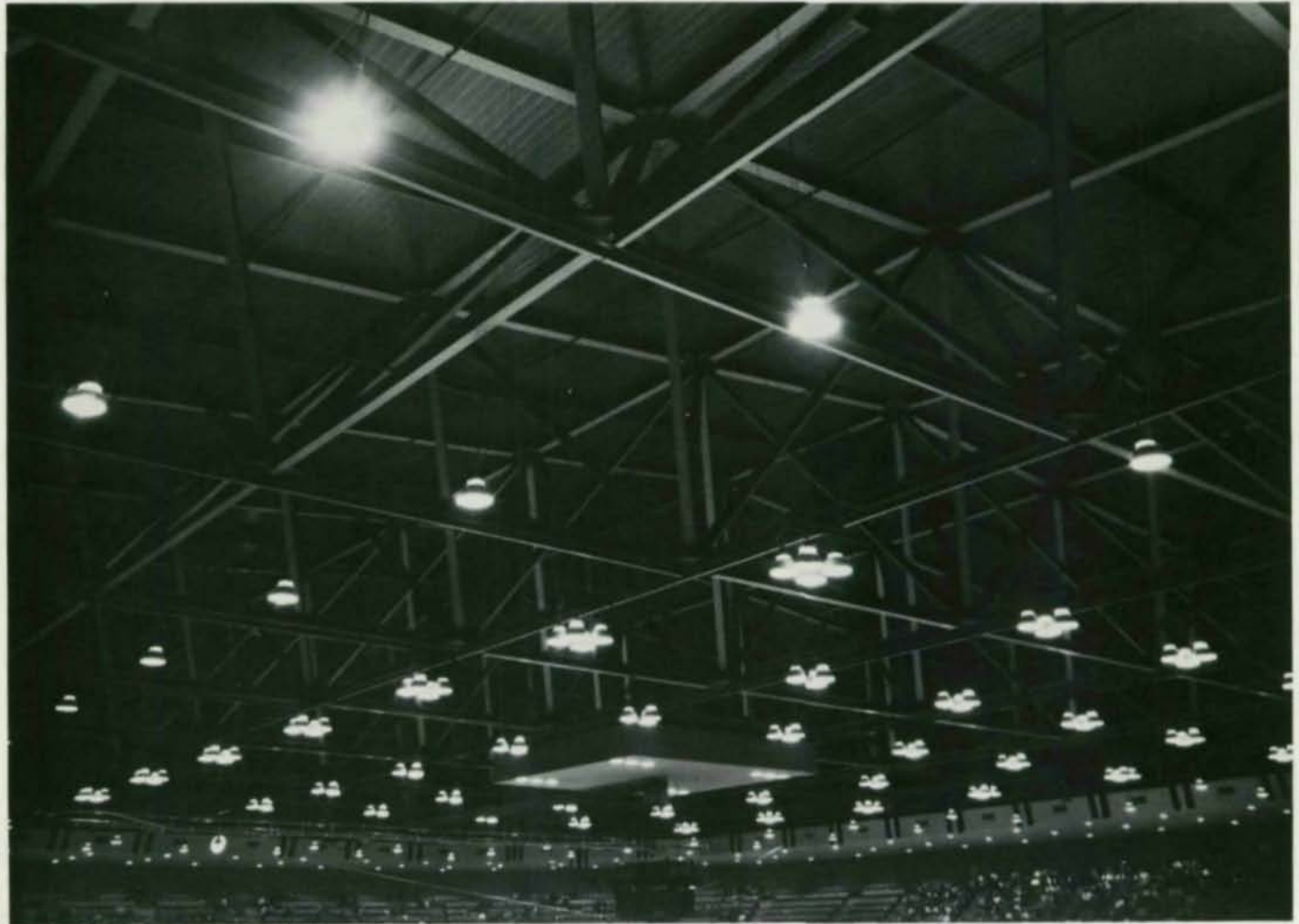
Arena lighting system is supported by exposed steel space frame 63 ft above floor.
