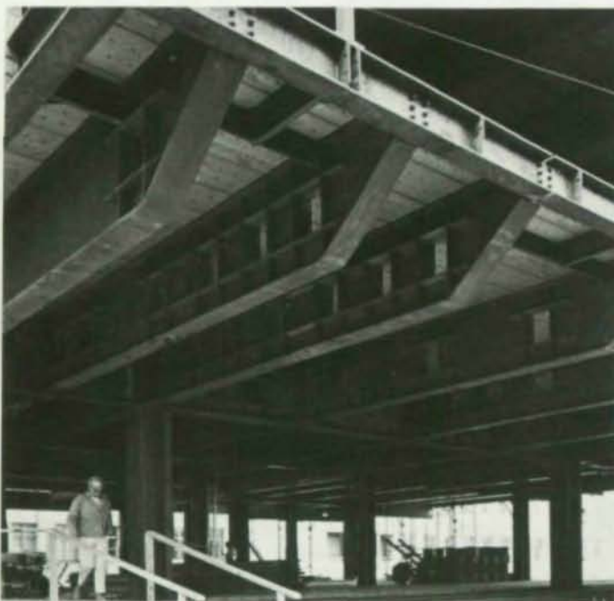
Cantilevered girders are 42-in. deep. Ductwork passes through stiffened web cutouts.
