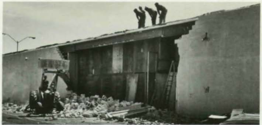
Tornado "blew out" walls on three sides of GES Department Store in Birmingham, but steel frame was undamaged.
