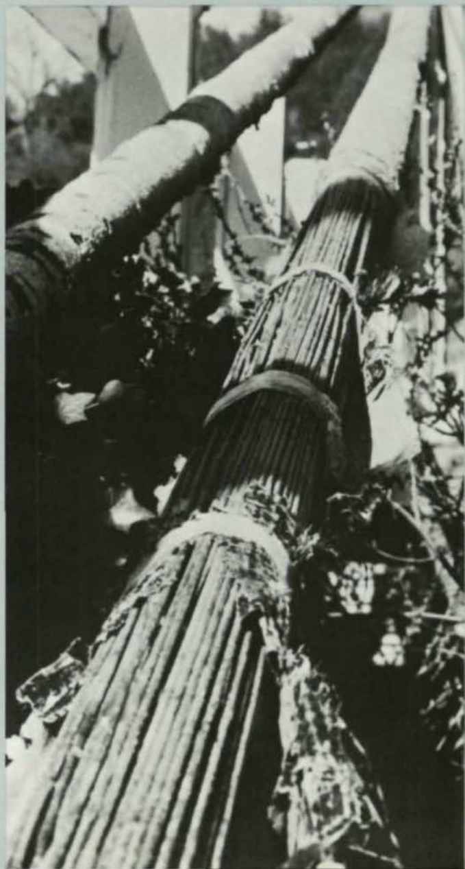
Cable covering deterioration near the anchorage. Exposed wires show little evidence of deterioration.
