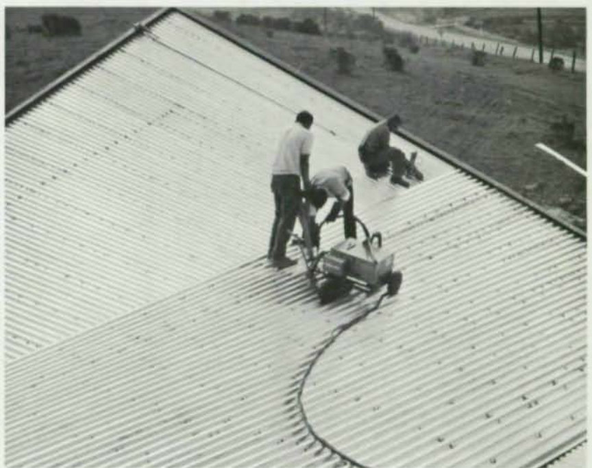
This economical hyperbolic-paraboloid roof is anchored at two low points 66.5 ft apart. Two layers of steel decking, laid at right angles and plug-welded together, are framed with steel edge beams to form the basic roof structure.
