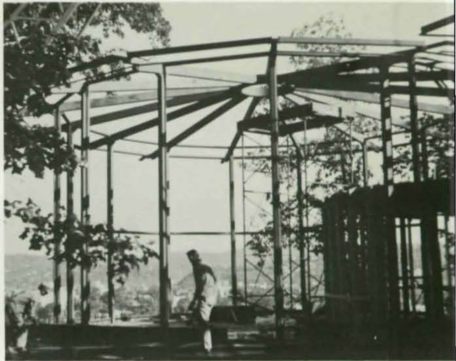
Lightweight tubular steel was chosen for the structural frame because it allowed the use of smaller members than could have been employed with any other material.
