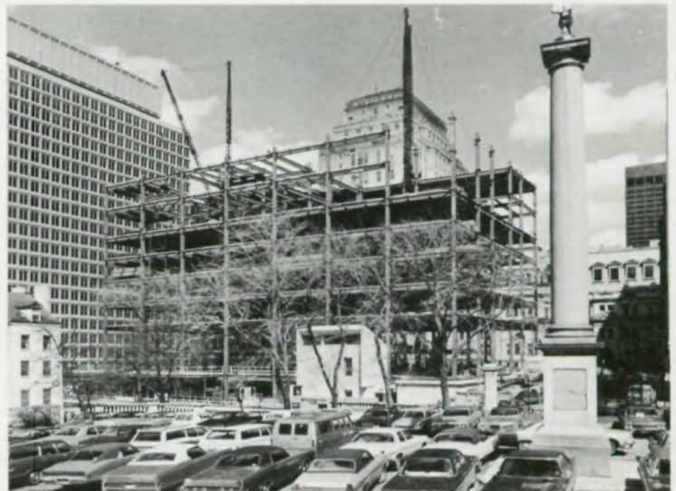
A588 steel was used for columns in the first three stories. The framework for the upper stories is A36 steel.
