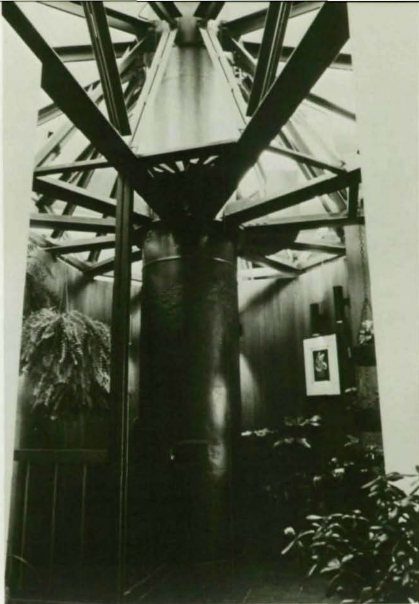
In the Portland, Ore., residence a circular steel column supports the structure.
