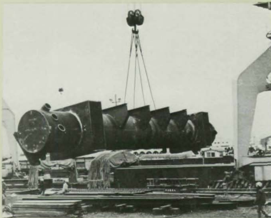
The tubular cable-anchor beam was shop fabricated with box girder and longitudinal stringer stubs in place.
