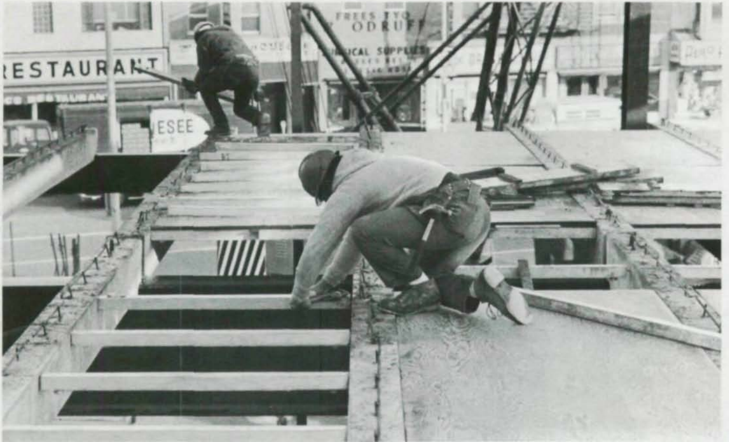
An inexpensive forming system of reusable standard plywood panels eliminates the need for intricate formwork and shoring.
