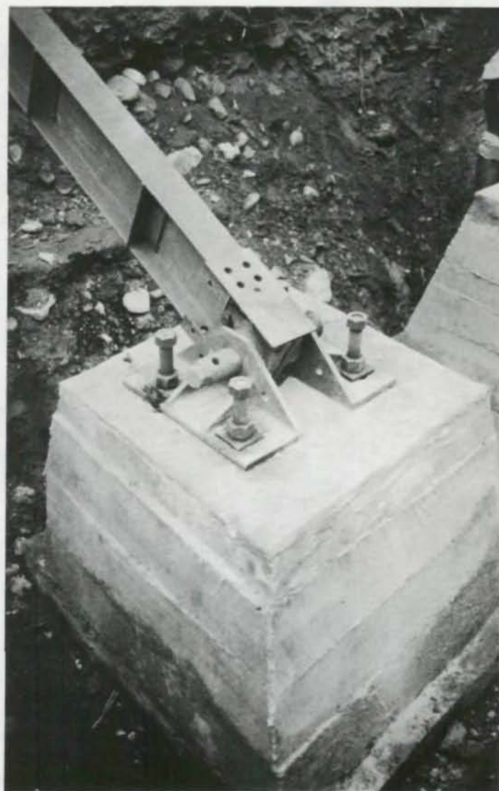
View of tower pin assembly, a motley collection of parts which were salvaged from junkyards and modified to fit in this configuration.
