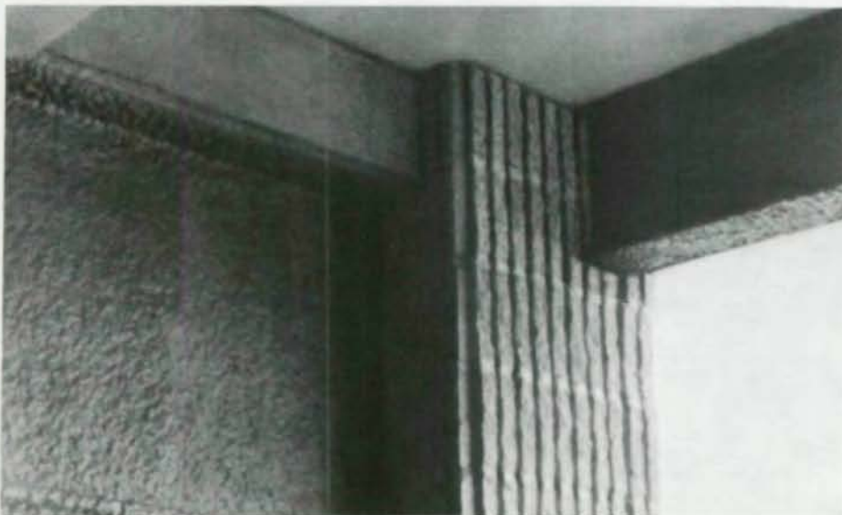
Girders and beams are fire-protected with a hard impact-resistant sprayed coating. Split-ribbed masonry block serves as fireproofing for exterior columns.
