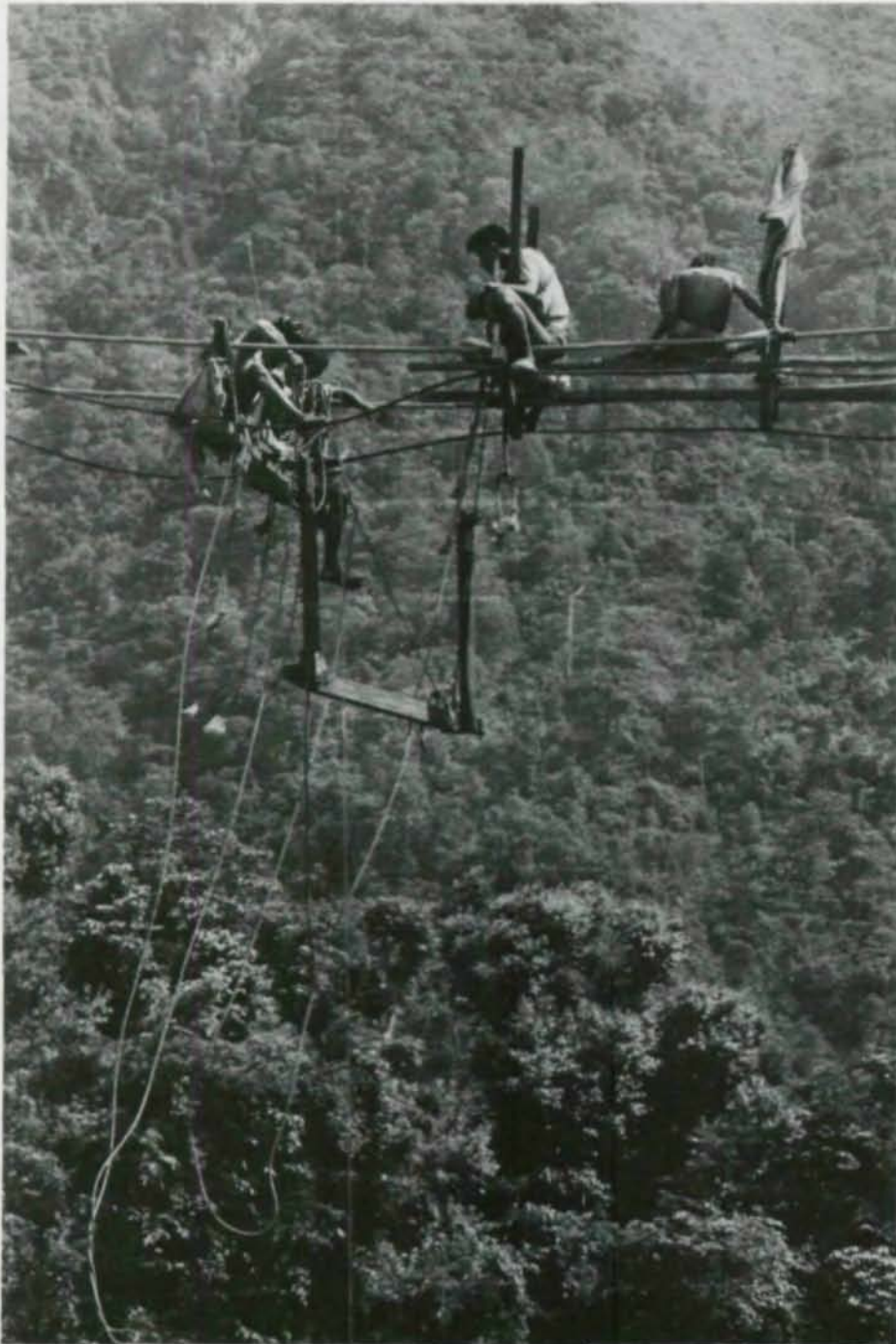
Perched precariously above the Kali Khola, workers hoist a "section" into place for the walkway.
