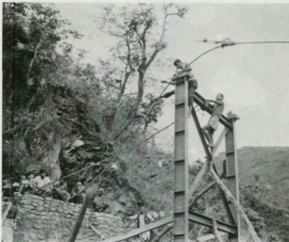
The main cable is clamped to the "saddle" at the top of the tower.
