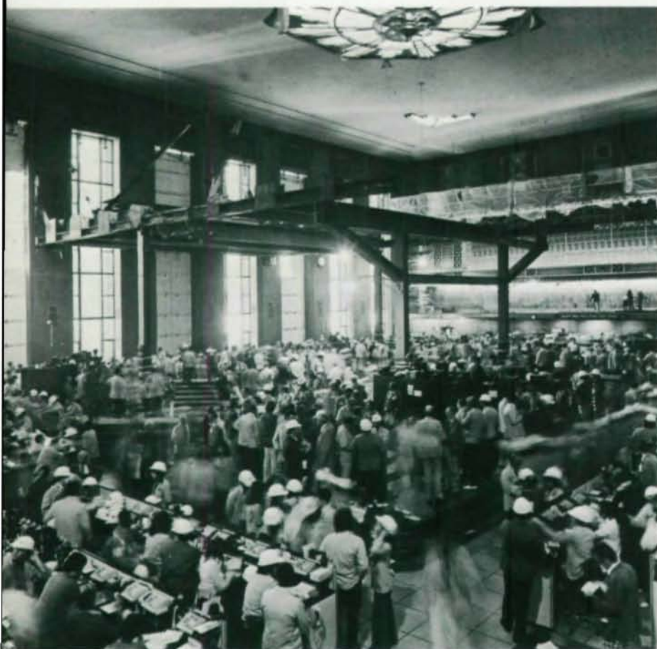
View of trading session under four temporary columns and bottom chords of the steel trusses
