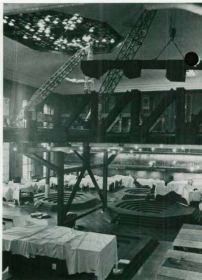
Top chord of one of the steel trusses being brought into position at night
