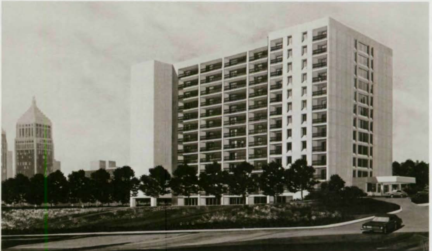
Fast steel erection made up for winter delays, put the project back on schedule.
