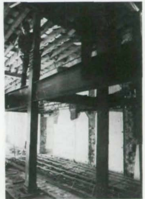
New steel columns (Task 3) given intermediate bracing by installation of new fourth floor (Task 6).
