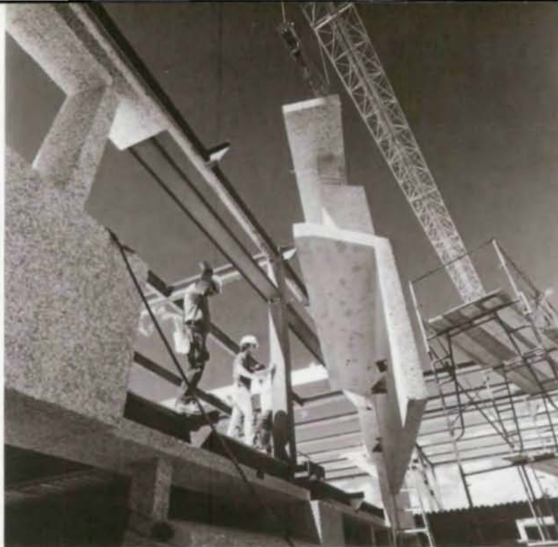
Precast panel with integrated shading device swings into place on steel frame.
