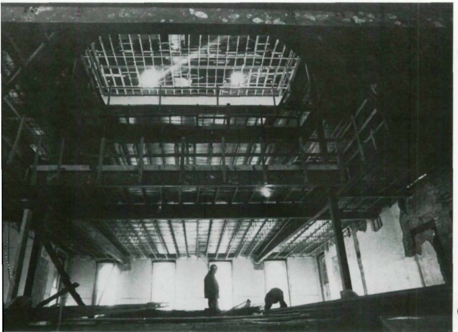
Looking up through atrium to added fifth floor ceiling from new second level.
