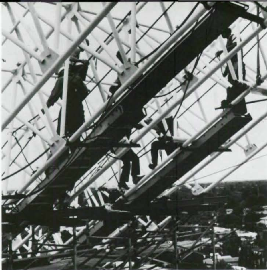
Lots of miles "climbing the iron" went into fitting assemblies of gigantic filigree of steel and glass.
