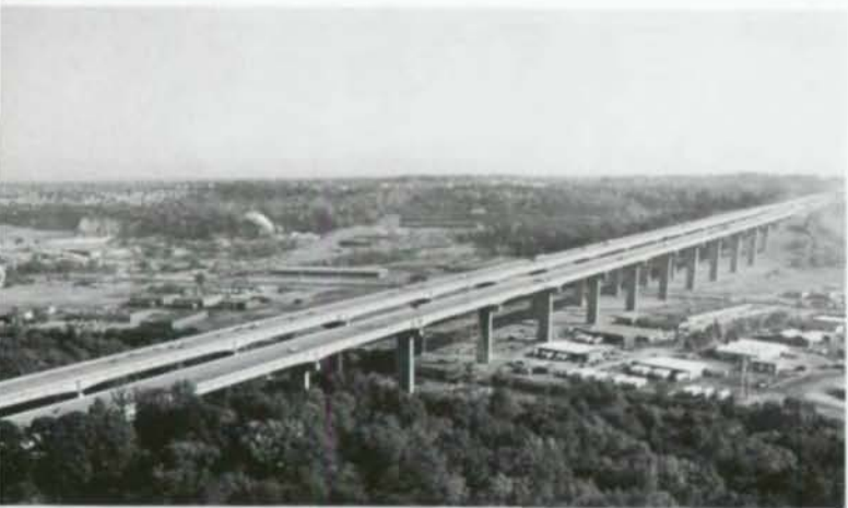
AWARD OF MERIT 1980 — ELEVATED HIGHWAYS OR VIADUCTS I-480 over Cuyahoga River Valley Cuyahoga County, Ohio
