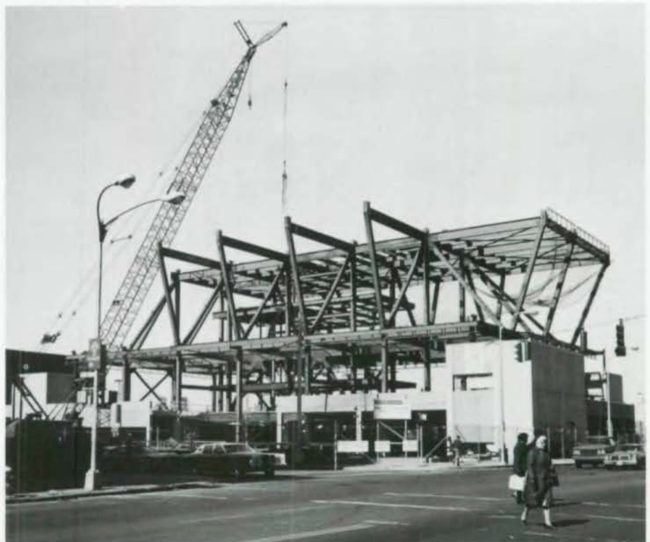
Exposed structural steel framing reveals crucial engineering of connections between existing and new columns (r., and below).
