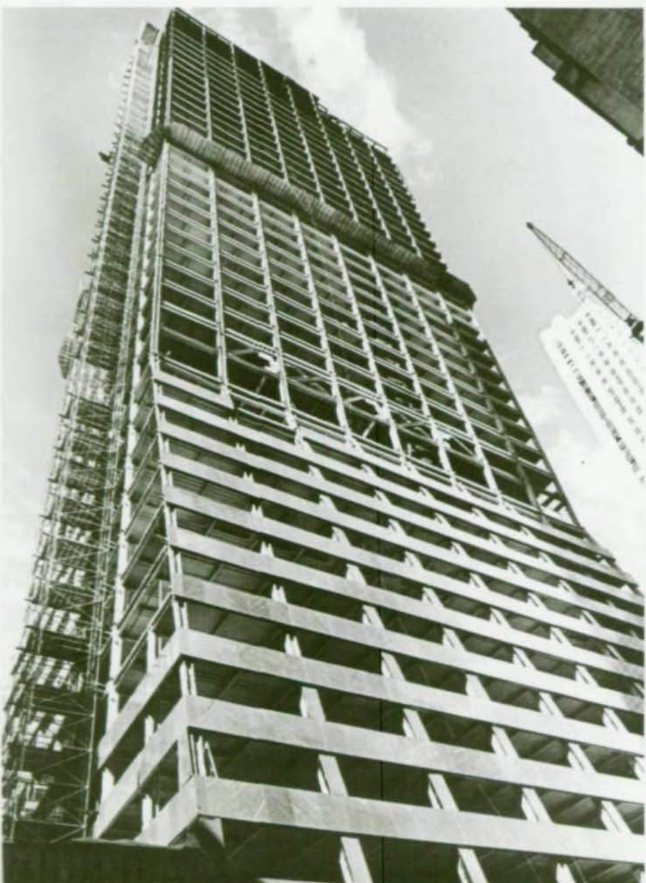
Structural steel goes up on 520 Madison Avenue Building in New York City.
