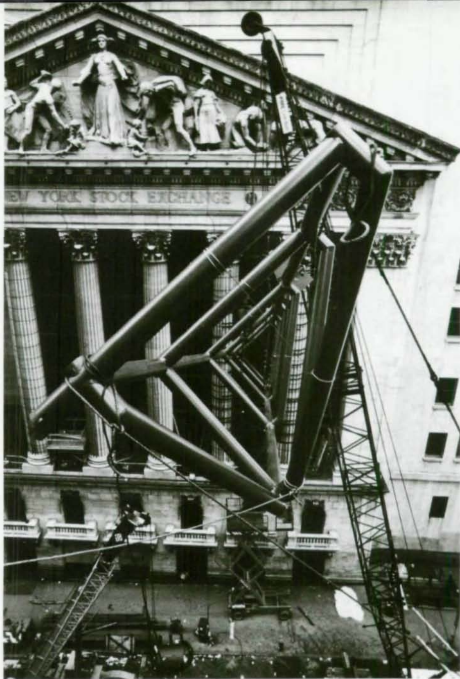
Tight squeeze. Two 18-ton trusses were prefabricated, shipped to site in sections, then wrestled between historic Corinthian columns through narrow windows (below) of New York Stock Exchange—all without disrupting business.
