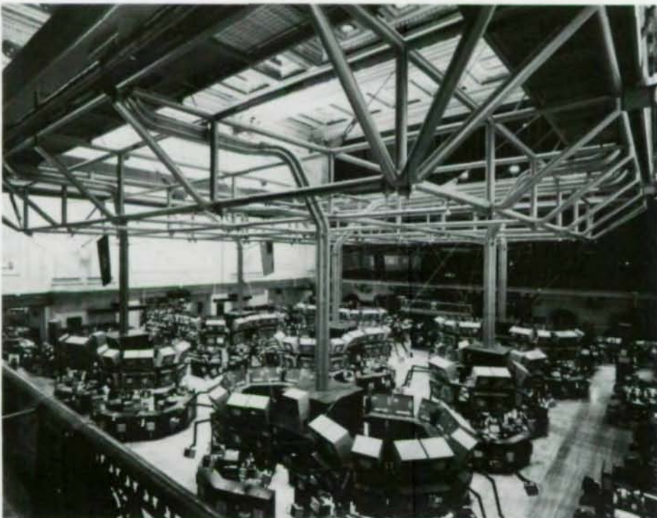
Steel space frames serve trading posts on remodeled New York Stock Exchange's main floor. Frames carry communications/cooling lines to sophisticated electronic equipment. Original trading floor shown (r.).
