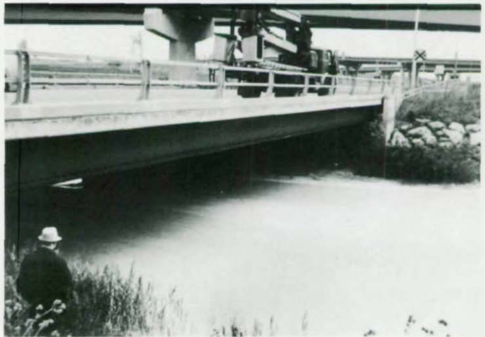
Nine Mile Creek Bridge, Syracuse, N.Y. is in industrial environment, with heavy salting and chemically polluted stream below.
