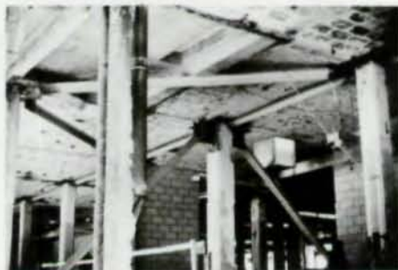
New horizontal diagonal bracing and existing barrel arch floors (top); and new horizontal and vertical diagonal bracing
