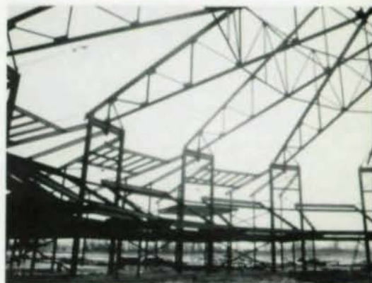
Structural steel roof trusses radiate from central core to create spectacular clear-span space.
