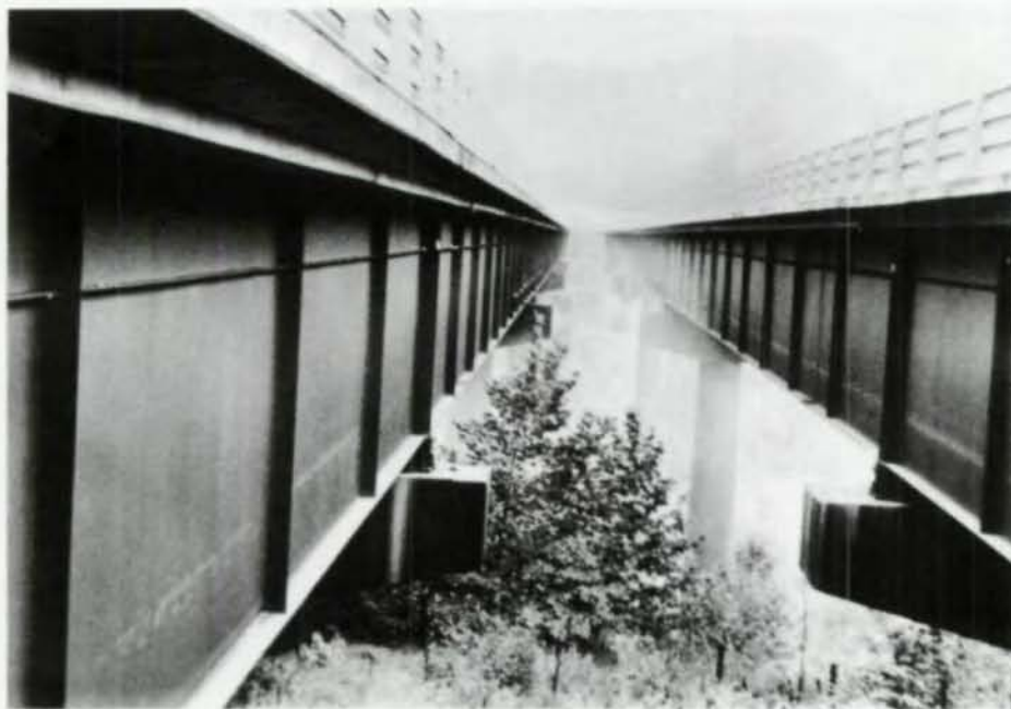
Structure, which carries I-26 over Green River (N.C.) is 12 years old. One of earliest bridges of weathering steel, and for years the longest span, it is subject to light traffic and salt conditions.
