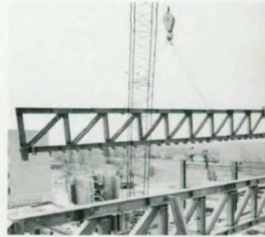
Giant trusses swing into place over existing hospital. Cantilever required loading each end at same time to avoid imbalance.
