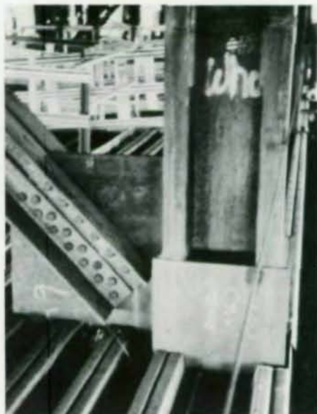
Diagonal bracing connection with core column
