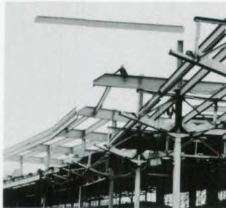
Trusses of existing roof were cut back 10 ft. New girders are W36x160. Bottom photo, new W12x20 column extensions support W21 beams and W36 girders that frame skyview box level.
