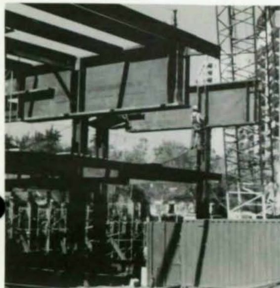
Massive steel girders move into place to provide both flexible floor planning above, and maximum parking arrangements below for luxurious structure's tenants.
