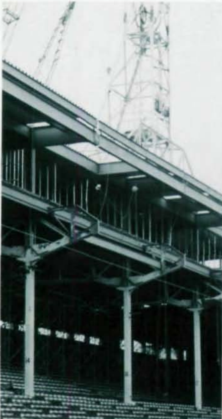
New steel framing for skyview box level erected above existing roof level.
