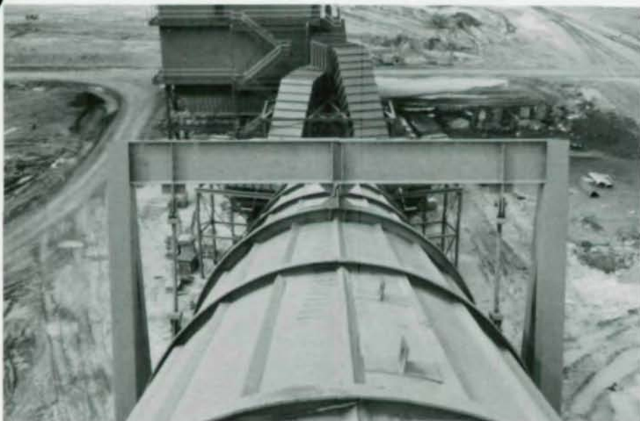
Figure 3. Front view of duct as it hangs hammock-style from 2½-in. dia. steel bars attached to top beam of supporting tower. Duct is welded cylindrical shell 3/16-in. thick, stiffened longitudinally by 20 3x3x½-in. steel angles. Transverse stiffening is WT6x13 rings 13 ft apart. At support towers, WT8x33 ring supports are used.
