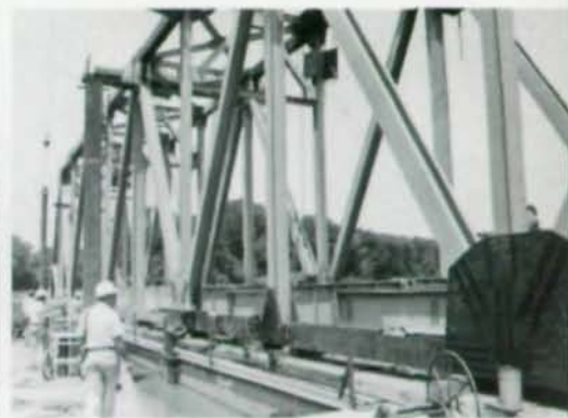
A BN-designed bridge was modified by removing 6 in. between each panel point.
