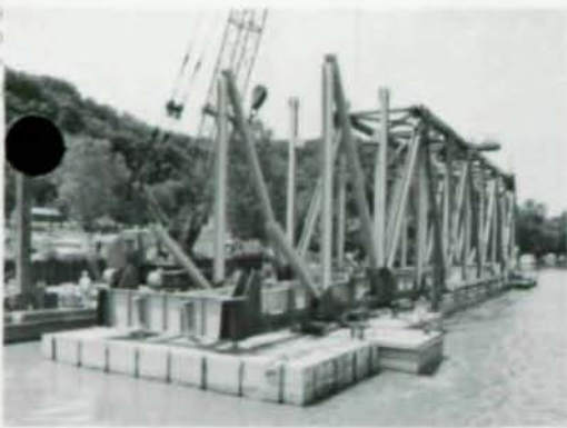
Truss span was field-erected on barges one mile north of bridge. Total erection time was eight working days.
