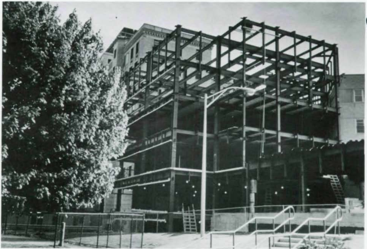
Steel framing of Northeast Building met most challenging structural problems in complex remodeling.
