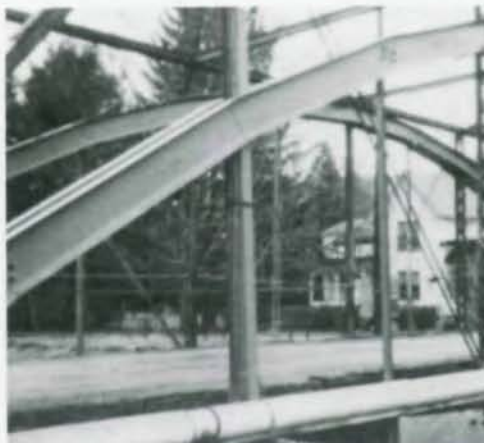
New life for rehabilitated 100-year old truss bridge at Coudersport, Pa. (below). Bridge can carry six times previous load limit. Closeup of new steel reinforcing arch (I.) that made it possible.
