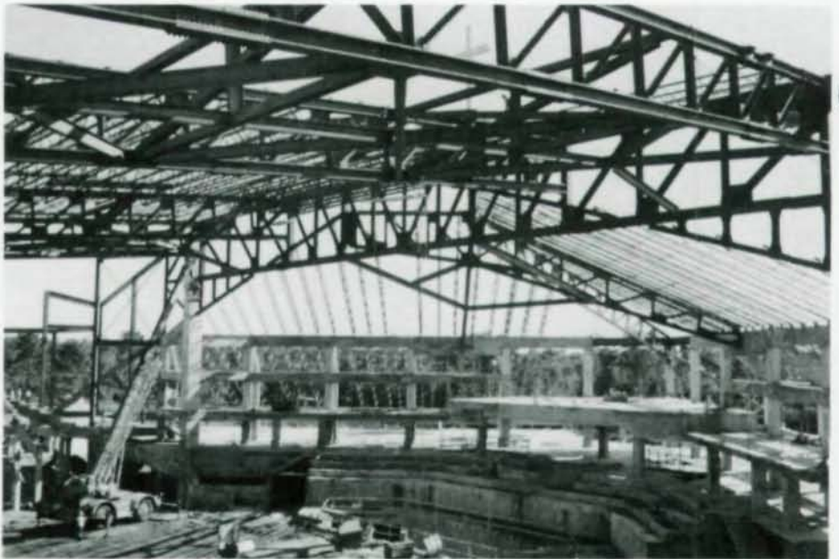
Main truss supports four secondary truss girders (av. span 174 ft). Two 80-ft long scissor trusses frame opposite side.
