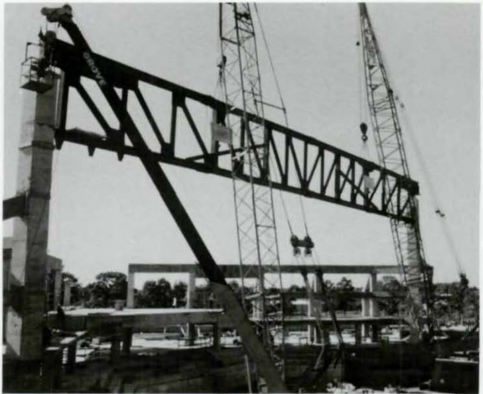
Main 180-ft long span in final position. Truss is 18 ft-6 in. top to bottom, with chords of W14x 426 A588 steel.
