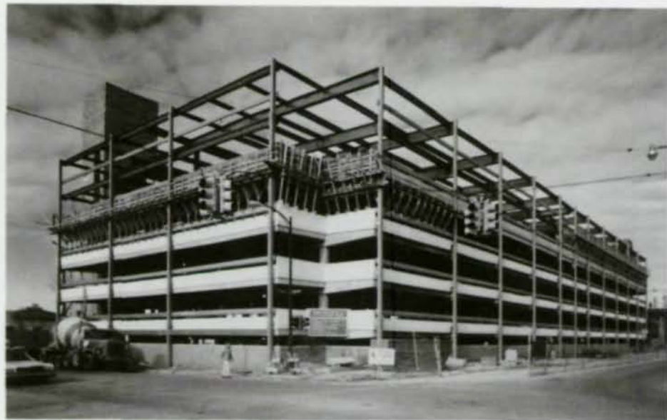
Ann Arbor, Mich. 3-level steel-framed addition straddles existing 492-car deck, provides 388 more spaces.
