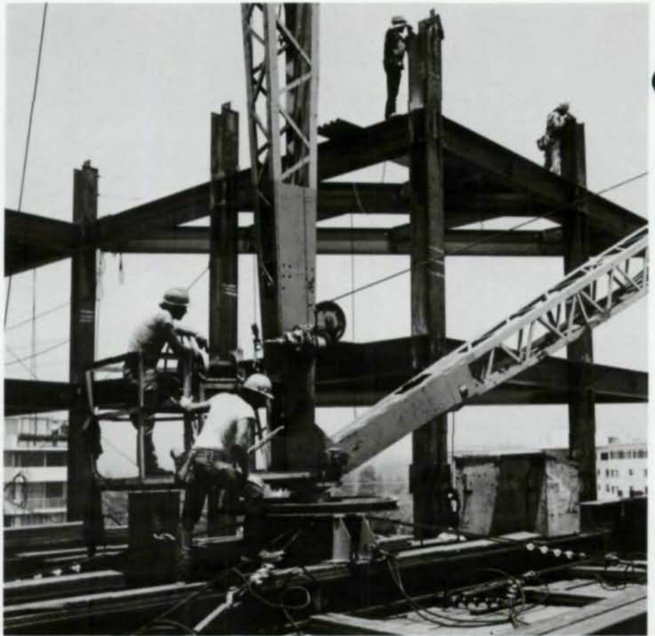
Steel-framed structure on fast track for time savings and flexibility for making changes.
