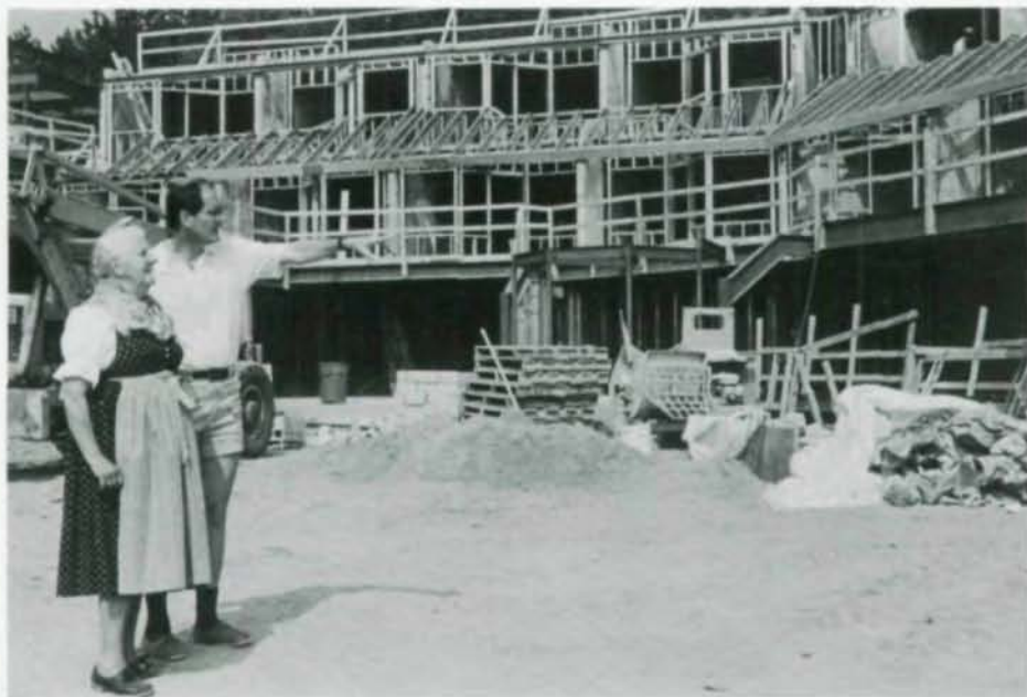
Maria von Trapp and son, Johannes, keep watchful eye on progress of new 73-room hotel.
