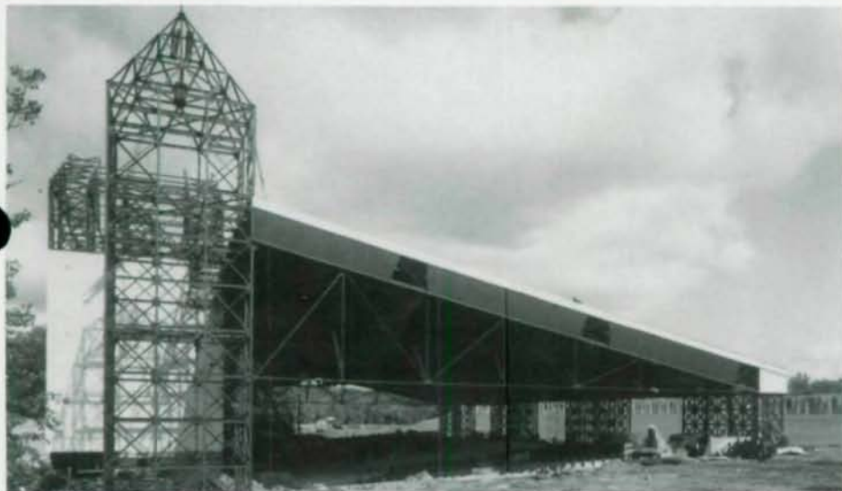
Open steel framework created web-like appearance for outdoor concert arena. Box truss between tower and playhouse supports trusses that cover seating area.
