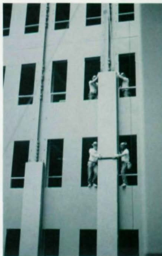
Column cover butts cover below and studs protrude through slots in panel. Note bolts at panel edges.
