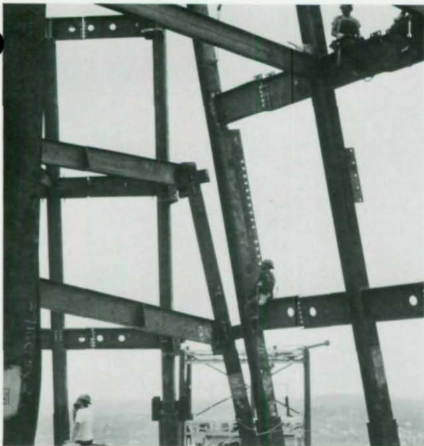
Direction of column trees at sloping top. Note fins for panel connections. Web holes give bolting access at panel horizontal joints.
