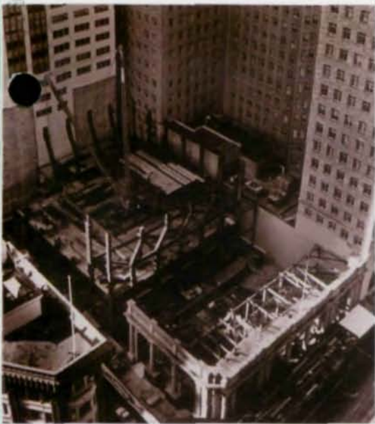
Start of steel erection. Sloping columns at 5th floor, and temporary bracing of existing bank's granite facade.
