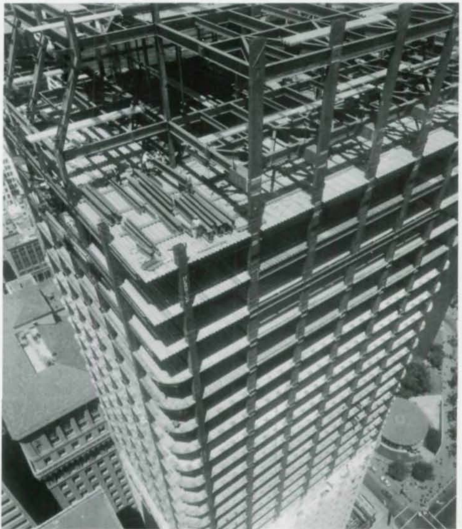
Top of steel framing with sloping columns at 42nd floor. Spandrel girders are recessed with torque box girders. Photo by Joe Perretti.
