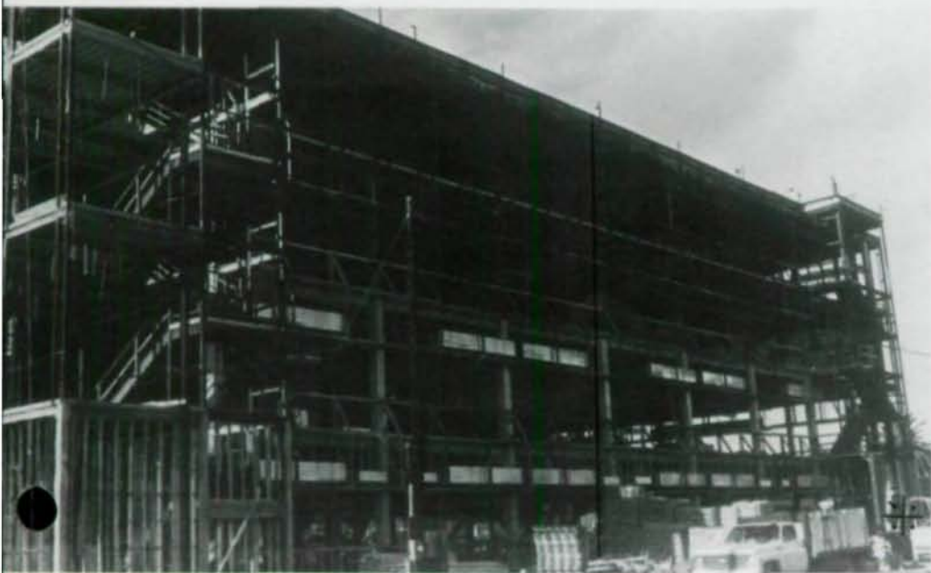
Structural steel framing met unusual demands for flexibility in present and future needs.
