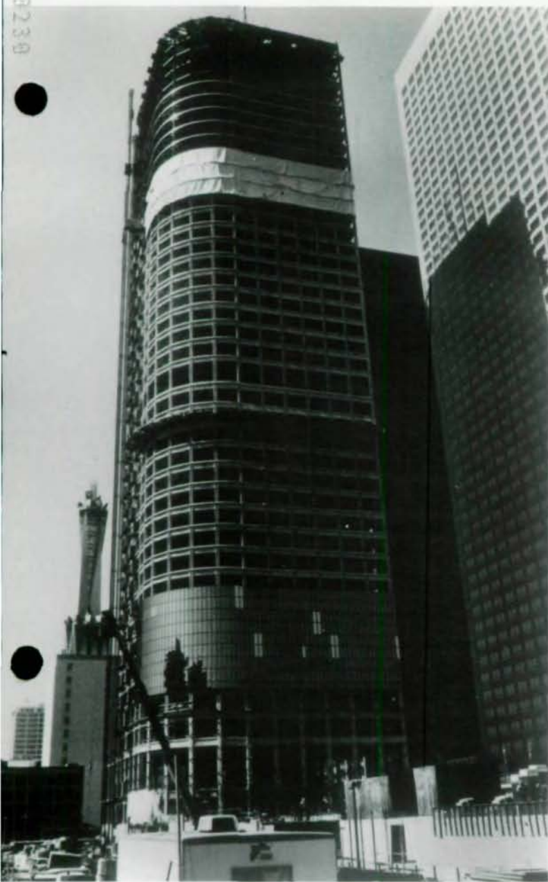
Highest point in downtown Los Angeles is graced by California Plaza (l.), focal point of first phase of huge $1.2-billion project. Tube-concept steel frame (above) withstands wind and seismic forces.
