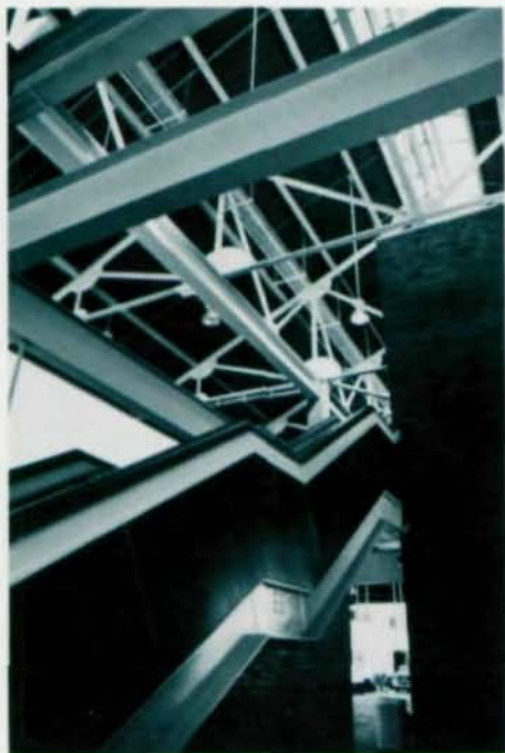
Steel framing was desired structural material for unusual gable roofs and numerous stairways and bridge spans.
