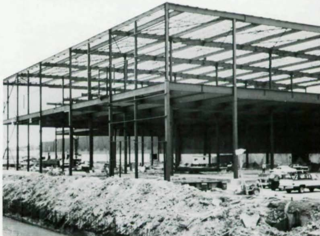
Primary Sort Facility —fast-tracking and steel framing (above) on Federal Express' new Memphis facilities made early occupancy a reality. Nearly completed structure is shown below.
