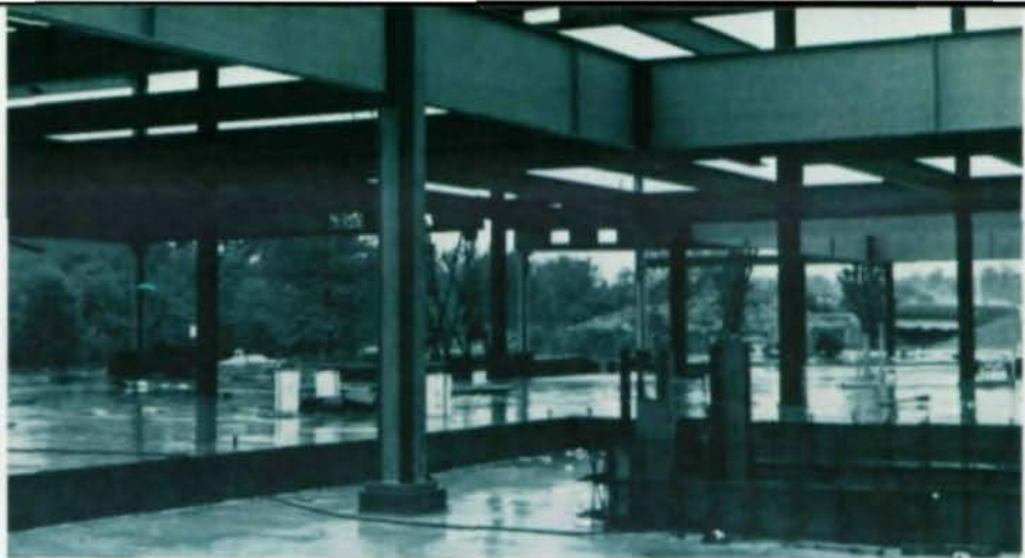
Common core elements, provided by steel framing, permit tenants greater flexibility in office planning.
