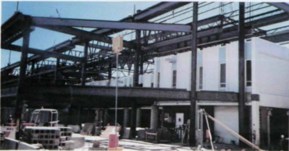
Existing structure was enveloped (above) by the new, using existing structure as work platform to construct new concourse and protect passengers. Enlarged concourse (l.) created by constructing steel superstructure around existing building.
