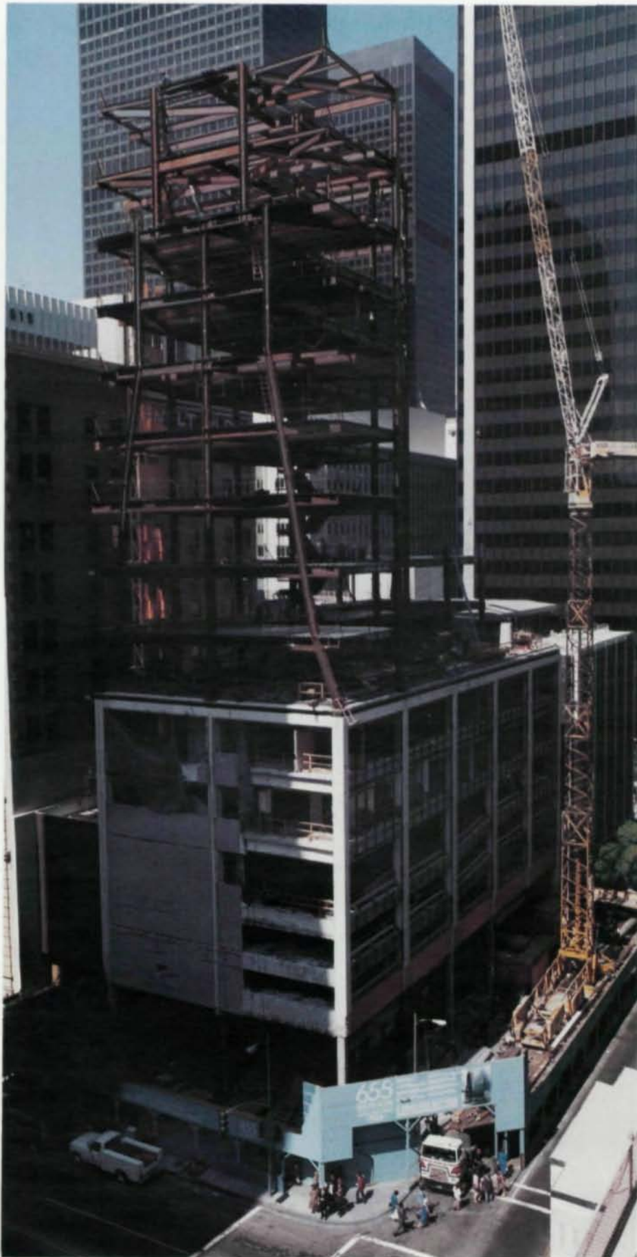
First for Los Angeles, a major renovation added floors to existing structure. Complex framing, plus tight site conditions, proved construction challenge.
