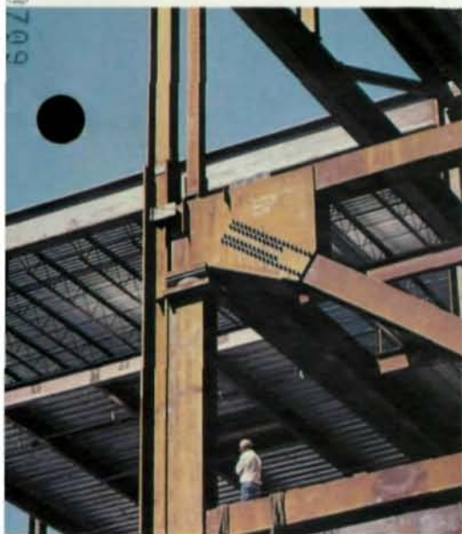
New structural steel tied addition to existing building. Project scheduling was critical to meeting deadlines.
