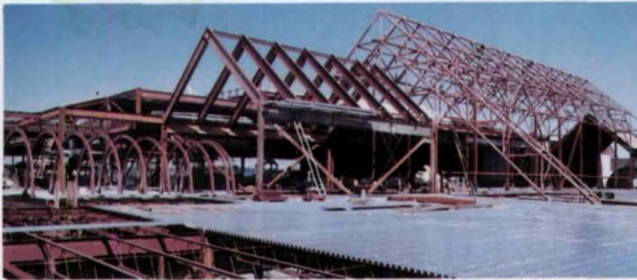
Three types of framing used to support roofs over lobbies. Barrel vaults employed over second-floor lobbies.
