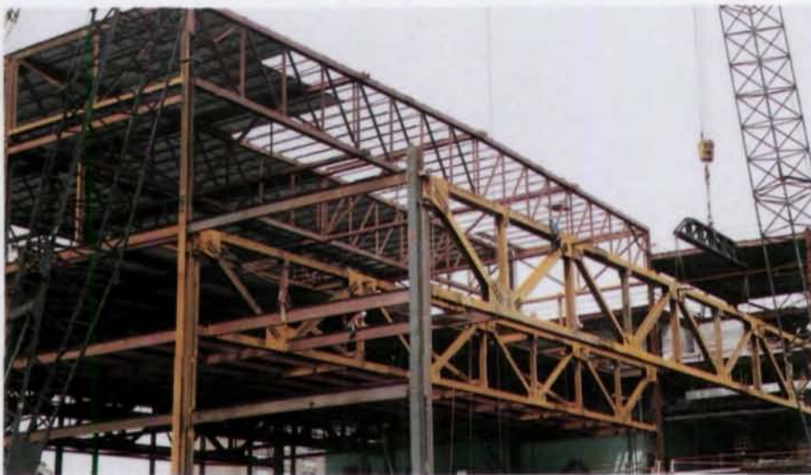
Deep (16-ft) roof trusses in existing building spanning 160-ft high bay area are double-angle sections with heavy angle chords.
