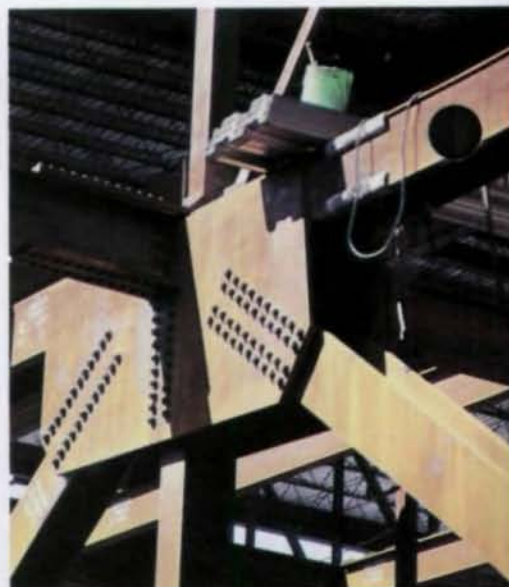
Gusset plates connect flanges of intersecting members. Trusses, weighing from 50-70 tons, were assembled on site.
