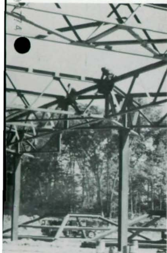
Trusses are connected into column pods in structural steel frame of TDC.
