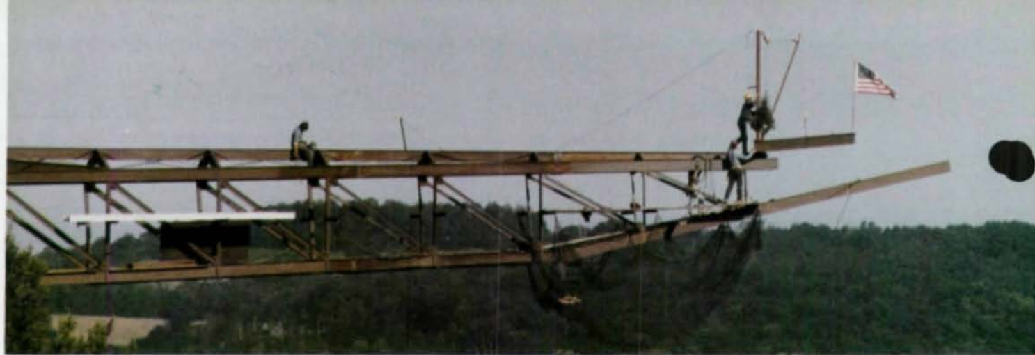
Tube of wide-flange sections carry cantilever moments of dramatic Infinity Room (above and r.).
