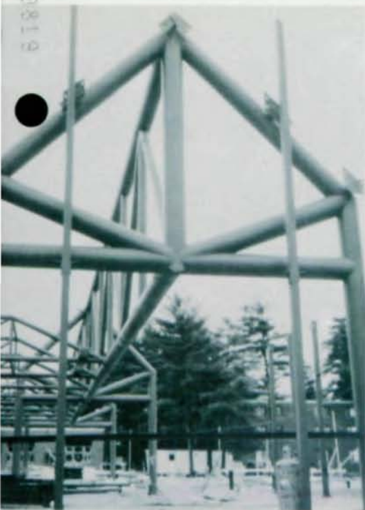
Column truss assembly permitted speed of fabrication/erection which made "dining in record time" possible.
