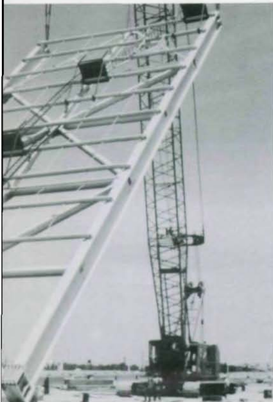
Two-truss assembly placed on column cap plates. Erection took less than 30 minutes.
