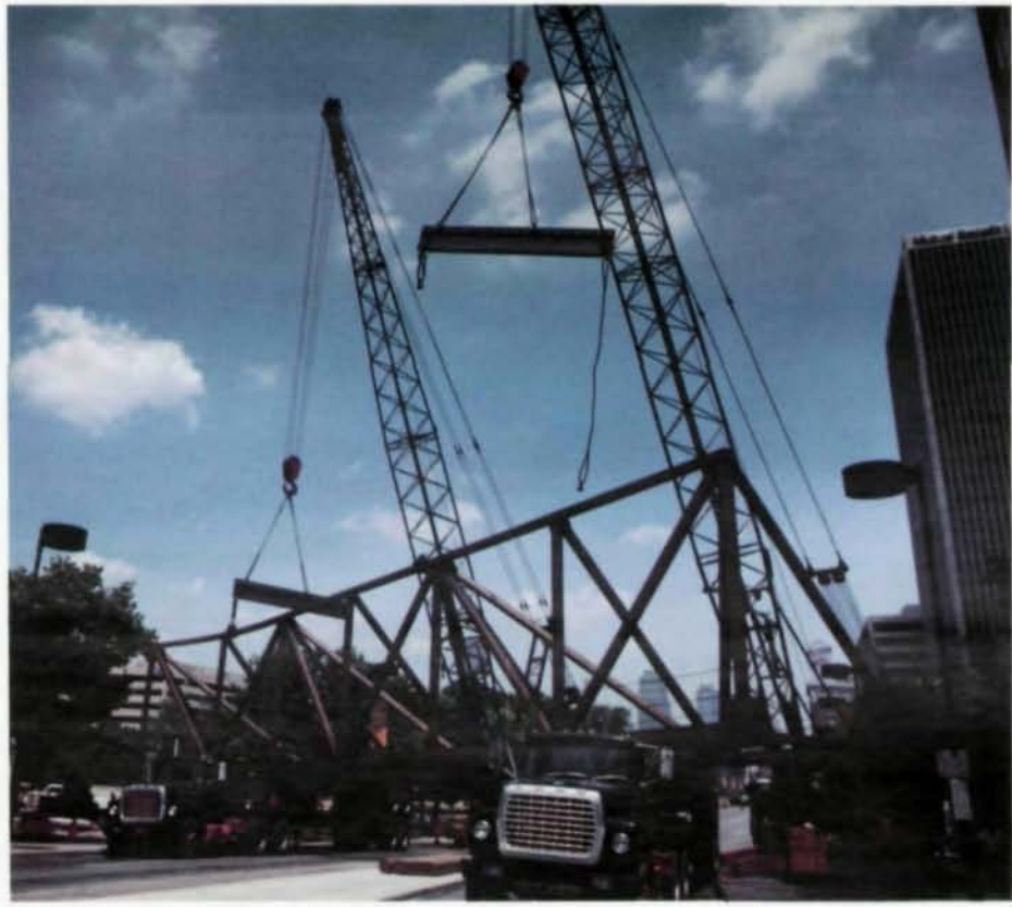
Half-span section of Westin walkway moves into position with two cranes and flatbed trucks.
