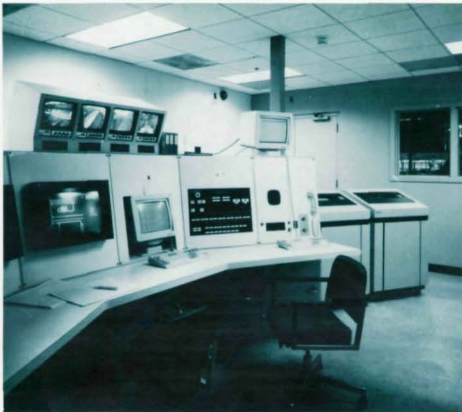
Operations in control room monitored by three computers in logic control system
