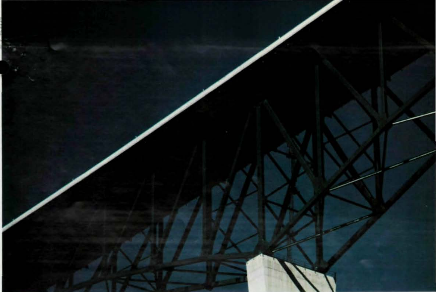
Steel design on gigantic bridge was selected in competition with a concrete alternative.
