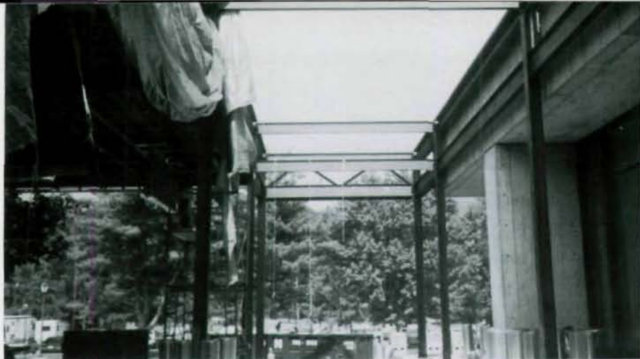
Looking down axis of atrium toward entry shows separation of skylight and existing building. Drawing (r.) details juncture.
