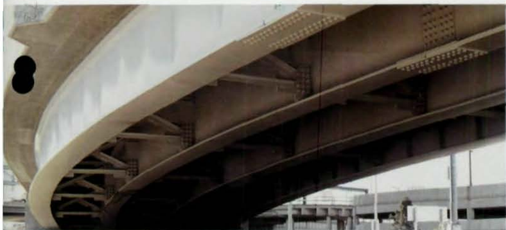
Sharp sweep of Ramp D girders (l. and above) show ingenious use of steel. Photo courtesy Delong's, Inc.
