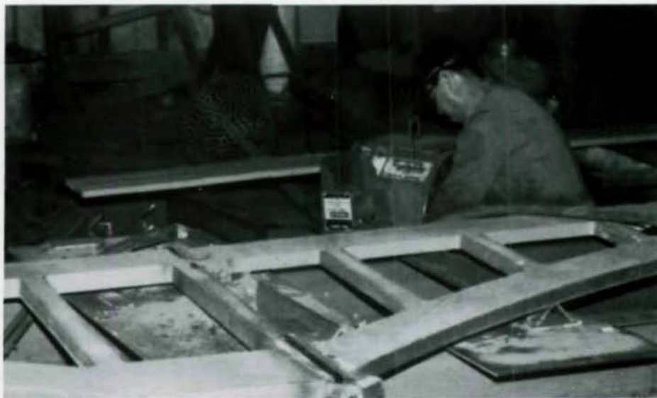
Closeup of single-web plate welded in fabricator's shop and pre-assembled into complete bridge.
