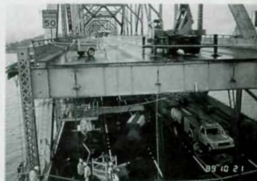
In contrast with the concrete Cypress section of the Nimitz Freeway, which will take more than three years to repair, the failed steel spans of the Bay Bridge were quickly replaced and the bridge opened to traffic just one month after the earthquake.
