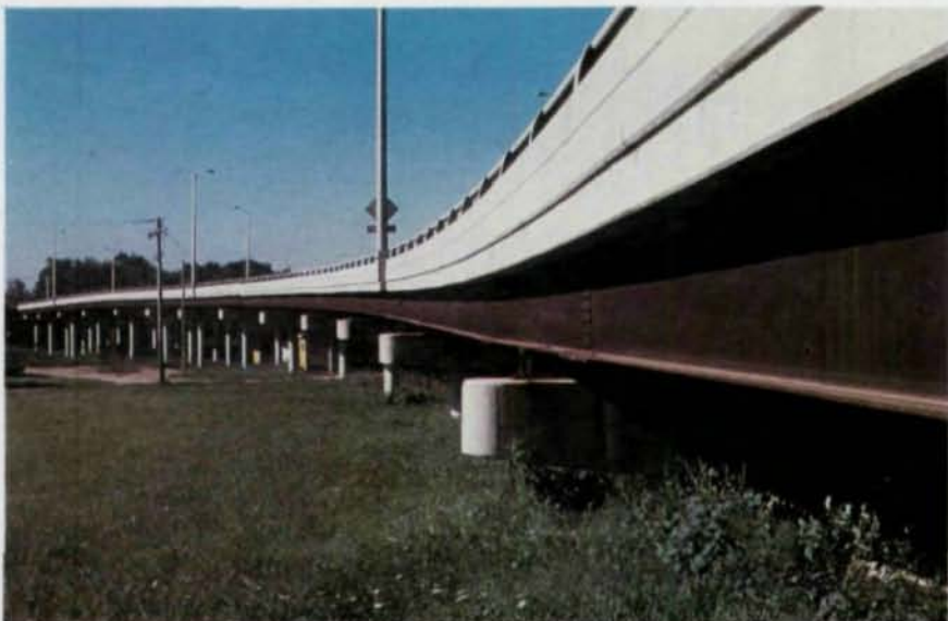
Weathering steel, when properly engineered, can often be used economically and without problems on a wide variety of structures. Shown above is a plate girder bridge.
