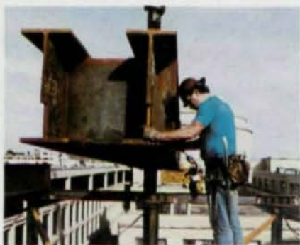
Pictured above is a closeup view of the large W36 x 300 girders as they were installed. The girders support hangers, which in turn support the floor slabs.
