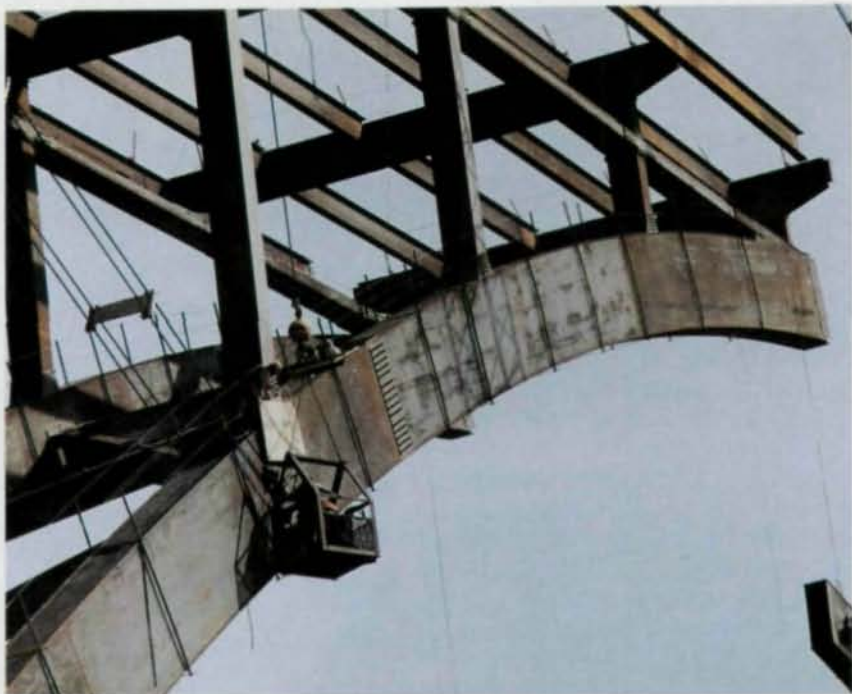
The arch ribs are a welded box section with internal diaphragms and stiffeners. The deck above the arches consists of welded plate girders placed transversely at 40' centers, and the stringers spanning between them were rolled steel sections.
