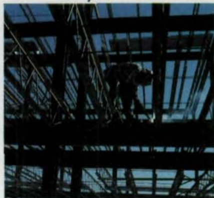
Lightweight Vulcraft steel joists were used in the Presbyterian Medical Tower in Charlotte, North Carolina.
