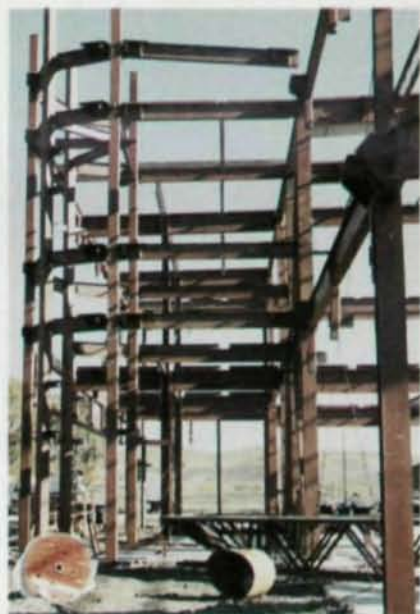
The rounded corners were created by placing small beams between the columns and hanging the precast cladding on the beams. The beam-column connections are provided by shear tabs welded to the columns and bolted to the beams.
