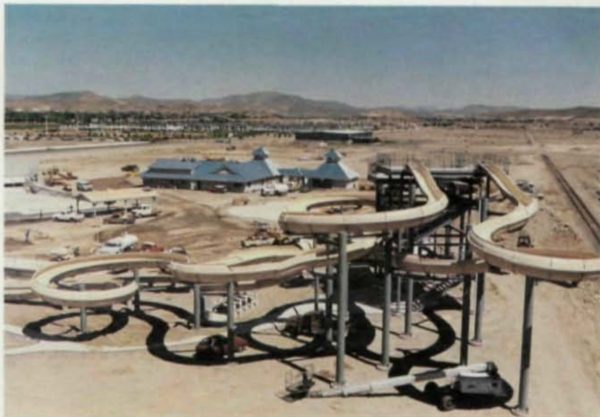
The water slides at Wild Waters used 200 tons of structural steel, including the 40' high stair tower. The support columns are clean shaft with a base plate at the bottom with stiffener fins. At the top is a closure cap so nothing goes down the column.
