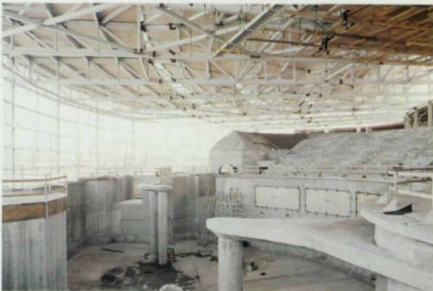
The Shedd Aquarium—inside and out. The largest of the habitats will hold two million gallons of salt water (top). Note that the steel trusses are still under construction. The addition's curving facade is a pleasing addition to Chicago's urban landscape. Top photo by McShane-Fleming Studios; bottom photo courtesy of Shedd Aquarium
