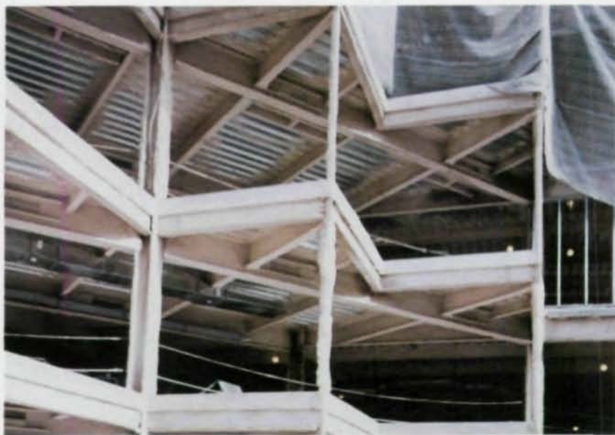
The framing over the main entrance needed to be cantilevered.
