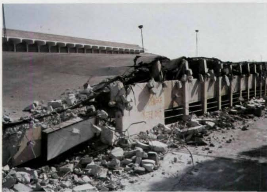
The magnitude 5.9 Whittier-Narrows Earthquake caused the collapse of the concrete parking structure pictured above, as well as several other concrete structures.
