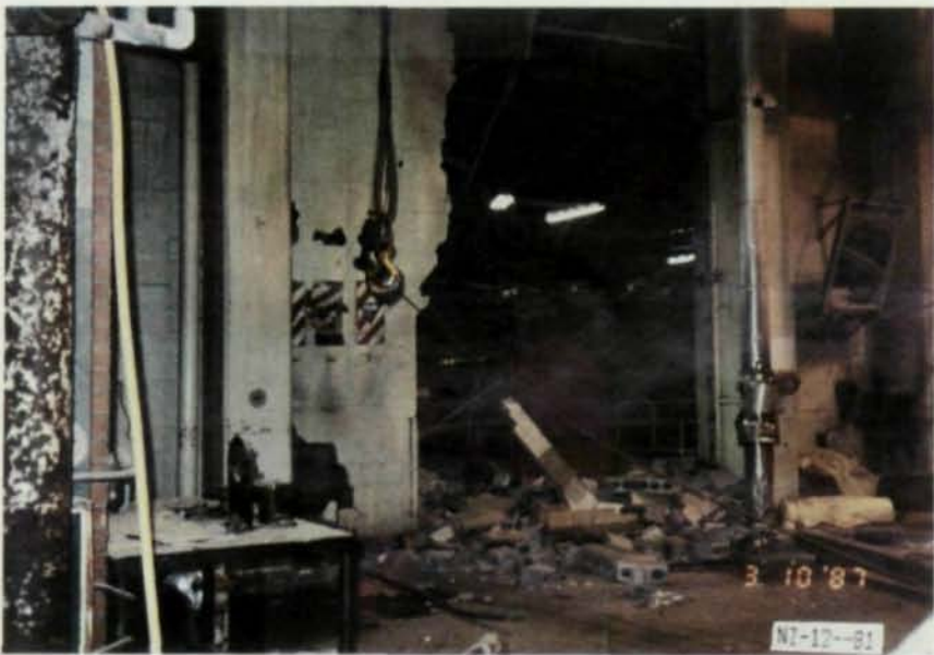
Typical mill building construction in New Zealand uses a high-bay, moment-resisting steel frame braced in the long direction. In the mill shown at top, the castellated beams framing the building experienced some permanent deformation. Pictured above is the Tasman mill, where several masonry walls collapsed, resulting in damage to the adjacent structures and equipment. As in the other mills, the steel was in good condition.
