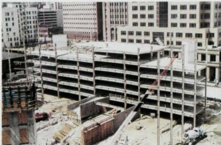
Construction of the seven-level 9th Street Parking Garage began in October 1989 and is expected to be completed in December 1990. The "skyway" connection shown in the model only will be built as needed.
