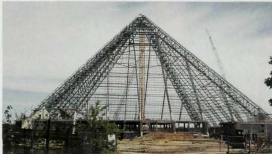
The Pyramid Arena in Memphis is a unique steel framed structure. Joists were used as part of the support system for the skin of the building.
