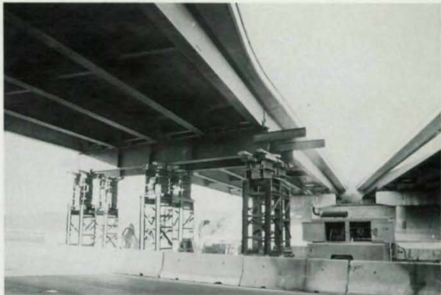
Two jacking towers were placed on each side of the three column locations to push the overpass back into position, which allowed four of the expressway's lanes to be reopened.
