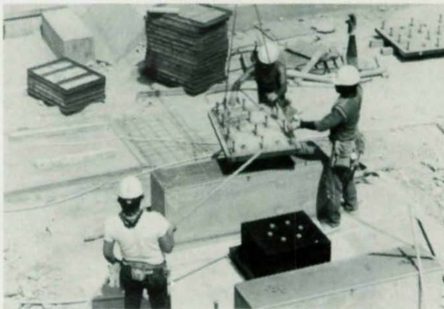
The base isolation system for the hospital at the USC Health Sciences Center in Los Angeles is designed to act as a "seismic shock absorber."
