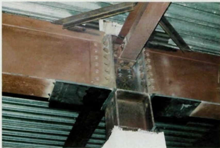
The existing beam-column moment connections (top) were shop riveted and high strength bolted in the field (above). Shear connections were made at the beam webs with double angles. The top and bottom beam flanges were bolted to the column flanges with split-beam tees. Shown is a beam-column connection at the eighth floor.
