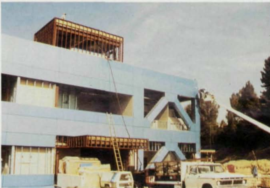
Above ground, the Fire Command and Control Facility for the County of Los Angeles Fire Department is a steel braced frame, while below grade it is supported on 32 base isolator units. The building's metal facade is designed to accentuate its structured elements.
