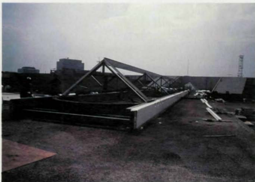
The renovation provides space for 100 additional shops, as well as two new anchor department stores (top photo by Hedrich-Blessing). The skylights are supported by 60'-long, W27x146 girders that were set in place by helicopter. These members are designed to support both the new skylights and the existing roof framing.
