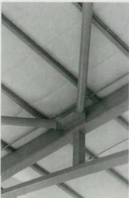
The top photo shows the top of a mill building column, including a crane girder supported off of a cantilevered tube bracket as well as an inverted single-span king post truss. The second photo shows roof framing with king post truss and rectangular tube purlins.
