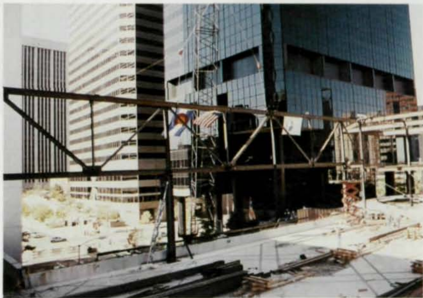
Steel erection was complicated by tight working conditions. Shown is the topping out of the new bridge trusses "piggybacking" the existing elevated pedestrian bridge.
