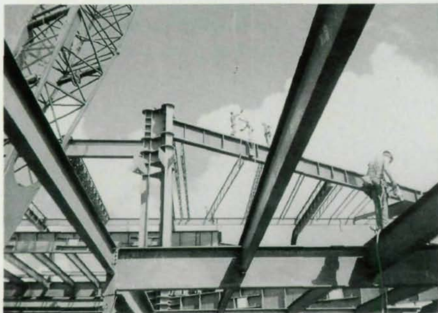
Delta's passengers are dazzled by the central hub, which includes a 12,750-sq.-ft. skylight covering a 140'-wide, column-free space. The massive skylight is supported on two compression rings, which, in turn, rest on 12 built-up tubes emerging from a series of cluster columns. Top photo by Steven Brooke
