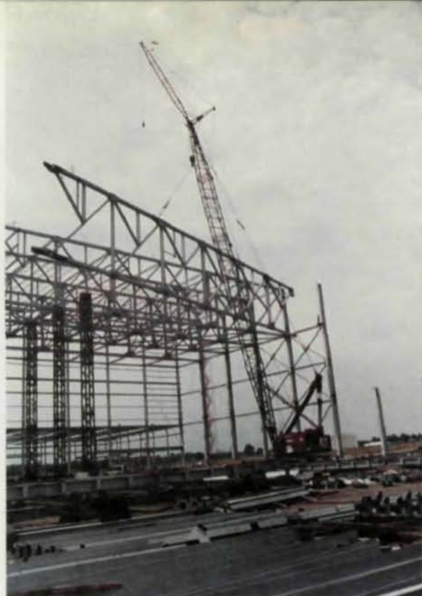
The hanger's structure consists of eight 412'-long Pratt trusses, with a depth of 26½' along the eave and 32' at the truss centerline.
