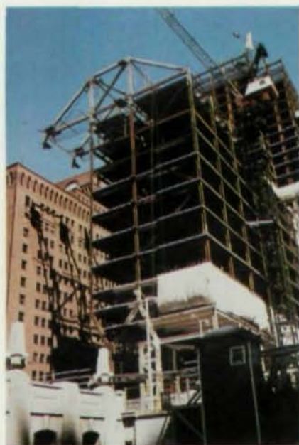
Shown above is the construction of the trusses and connections. Photo by McShane & Fleming Studio
