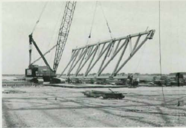
End sections of the truss were set at the columns by simultaneously lowering the top chord detail onto the column cap plate while guiding the truss bottom chord end member inside connecting gusset plates on the W36 column.
